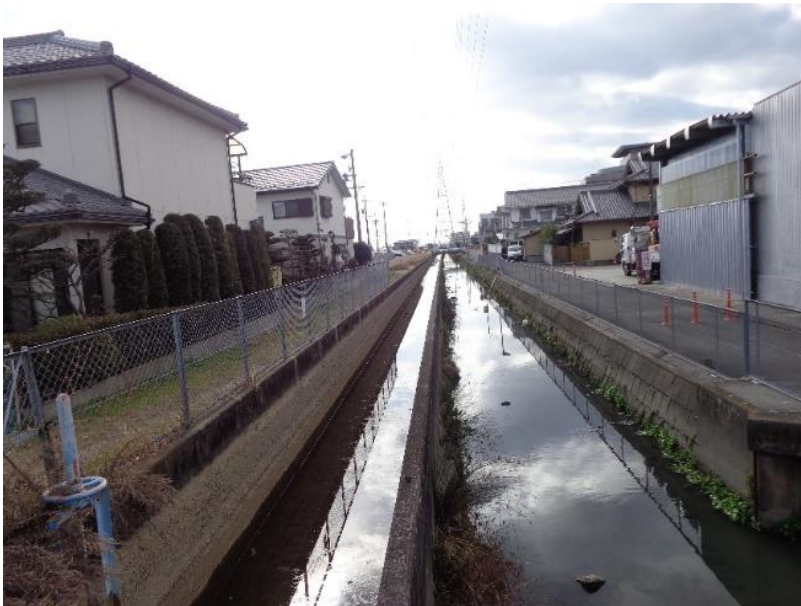
Figure 7.8 Open channel storm drain in Tsushima
