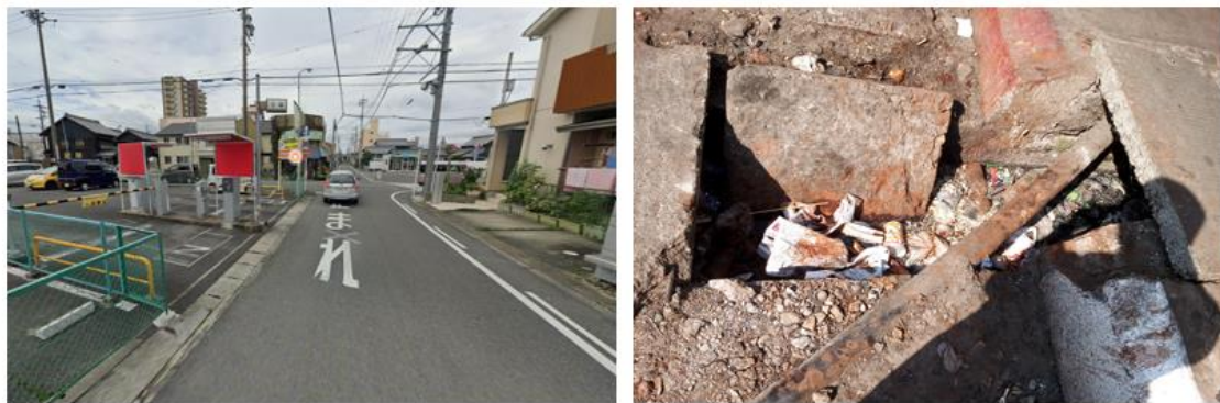
Figure 7.6 Storm drain with cover in Tsushima (left) and storm drain with no cover in Yangon (right)
