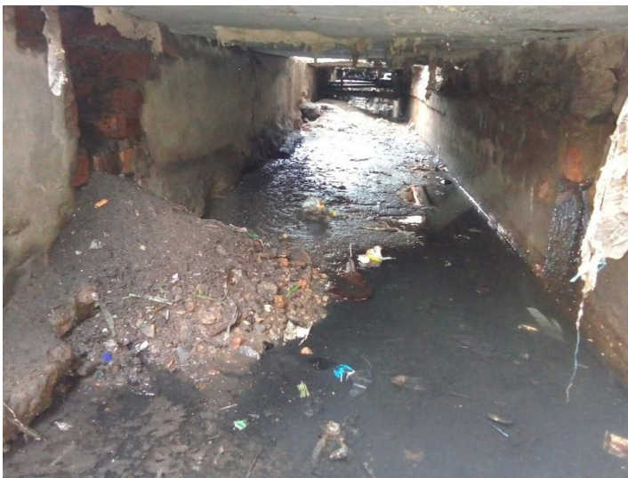
Figure 3.2 Sediment in the drain (source-DWMA Latha)
