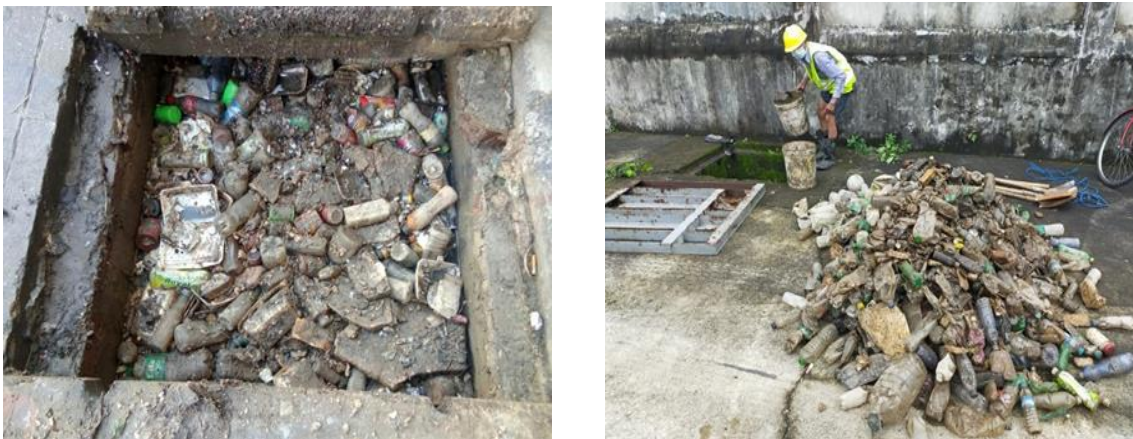
Figure 2.4 Waste blocking the drain in Yangon (Source-DWMA Latha office)
