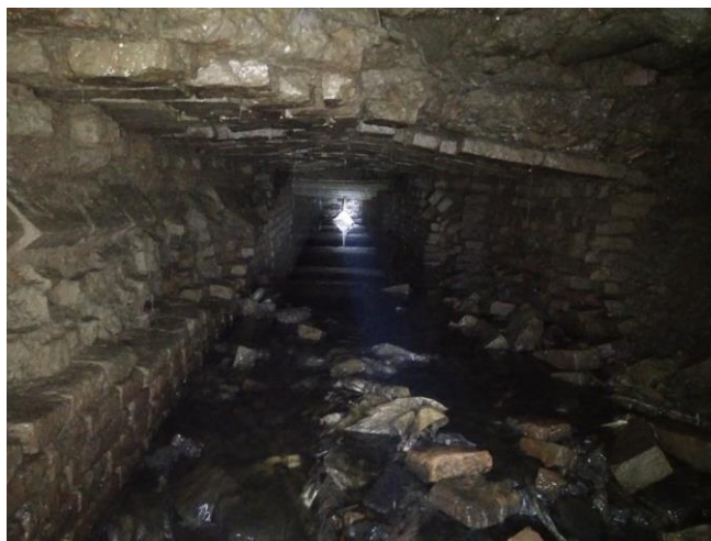
Figure 2.3 Structural deterioration of storm drainage in Yangon (Source-DWMA Latha)
