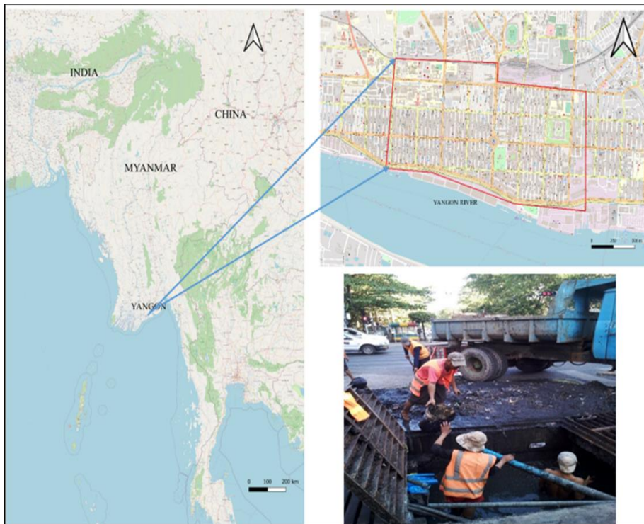
Figure 3.1 Location of study area and sediment dredging from storm drain in Yangon (map source: Open Street Map)
