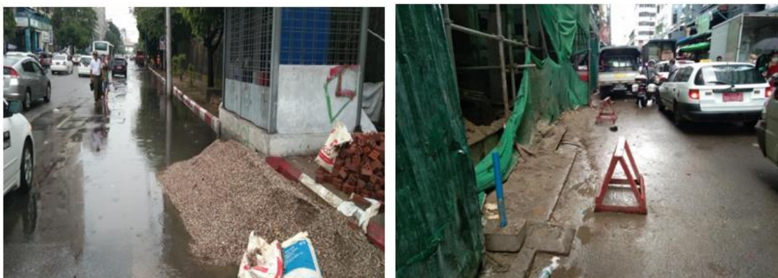
Figure 7.11 Construction materials, gravel and sand at the rear of drainage throats (source-DWA Latha)
