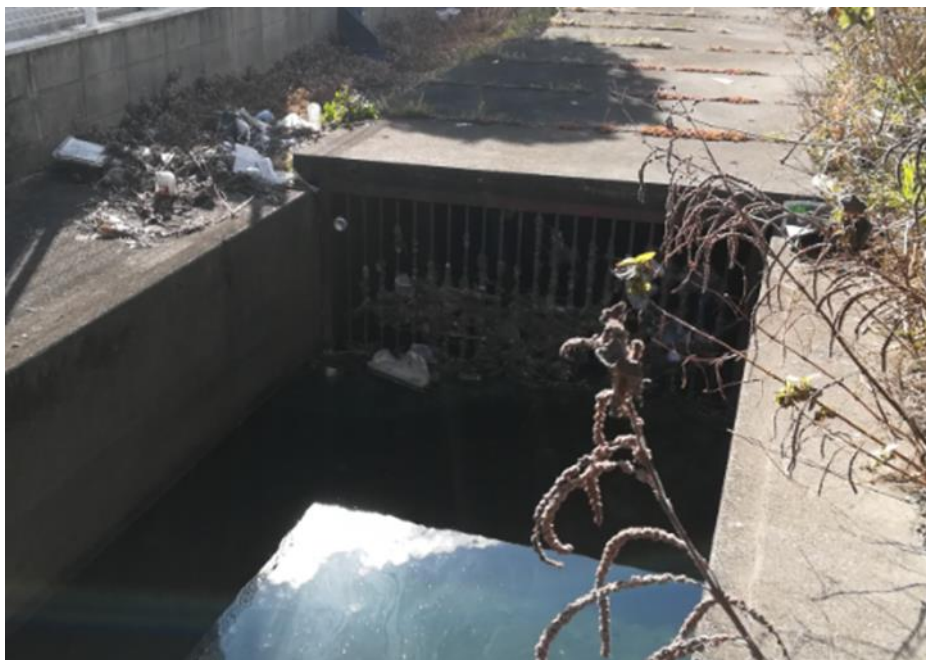
Figure 5.8 Garbage and organic debris at the trash screen
